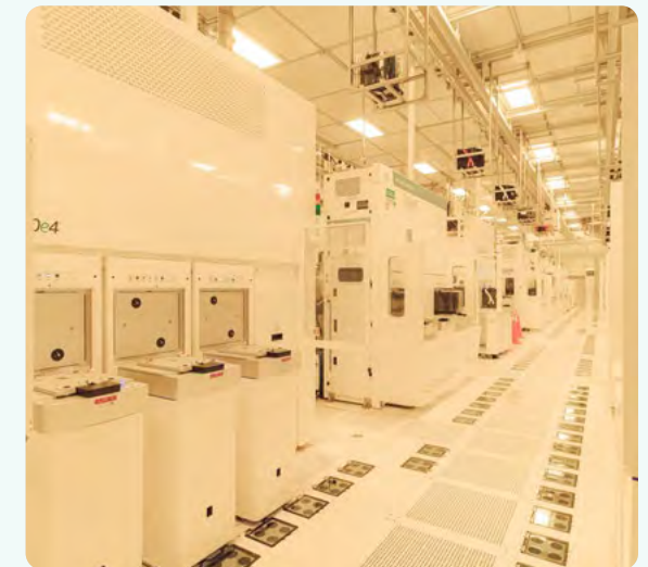
TSMC improves the structure of fans for dust-free rooms to improve energy conservation benefits.
