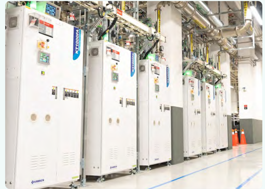
TSMC works closely with suppliers to renovate electric-heating local scrubbers to improve the reduction rate of N 2 O.
