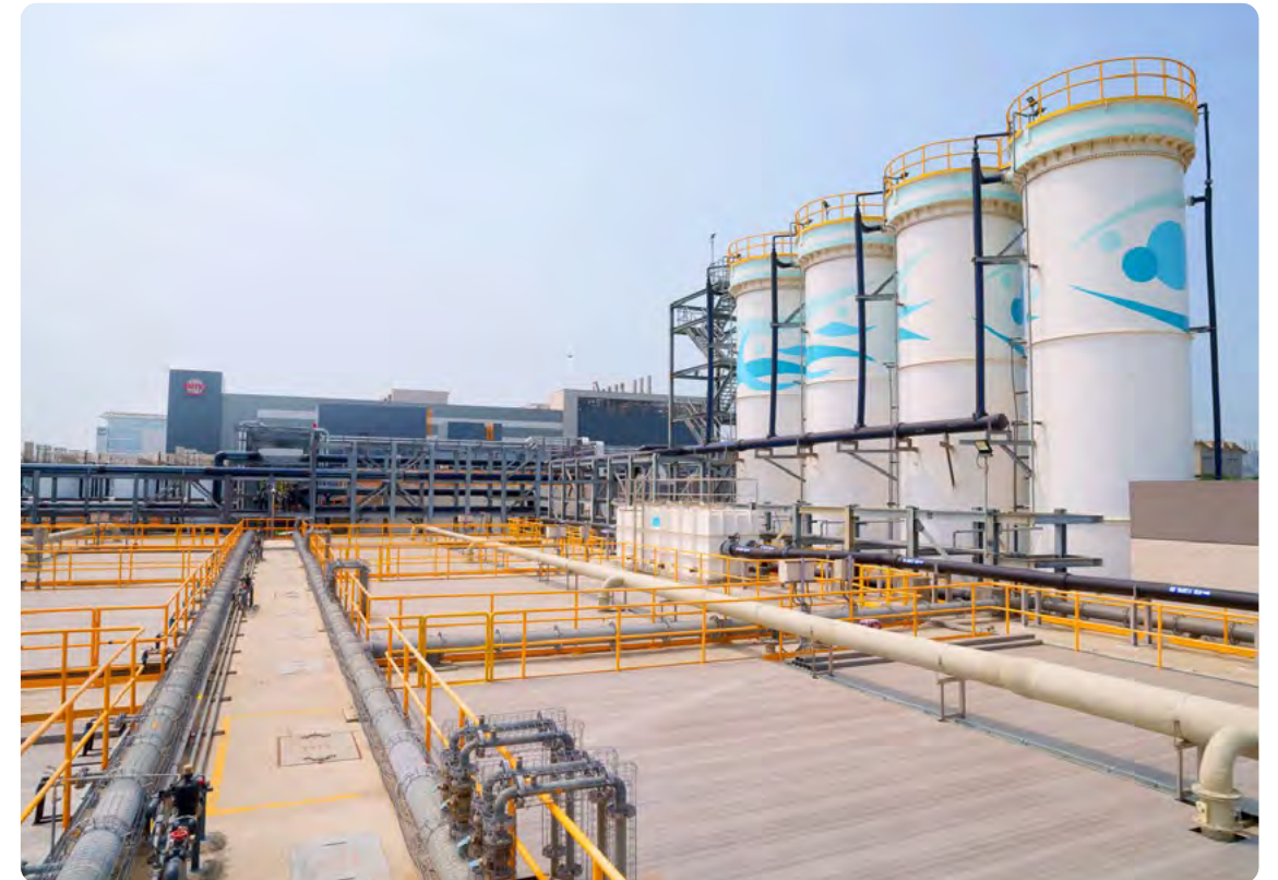
TSMC S.T.S.P. Reclaimed Water Plant
